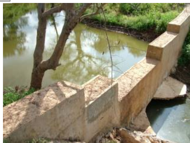
Sections of the apron have been undermined due to foundation and size of the apron being inadequate.
