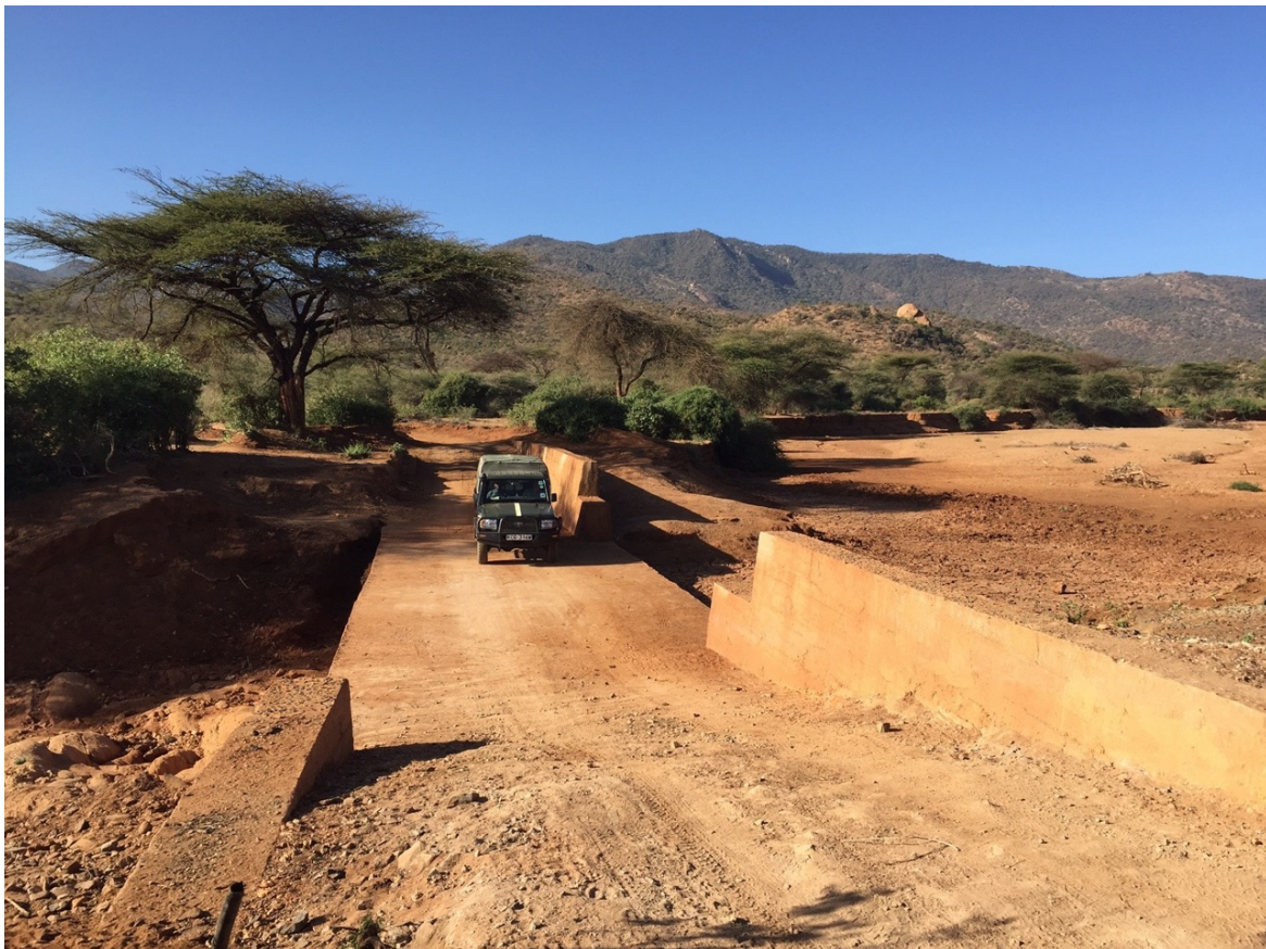
Sand dam road crossing in Lekurruki Conservancy, Laikipia, Jan 2017. [Photo Credit: David R Jordan.]
