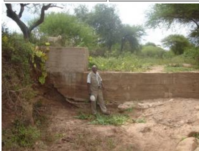
Erosion of left hand bank shows the foundation and apron do not extend into the riverbanks
